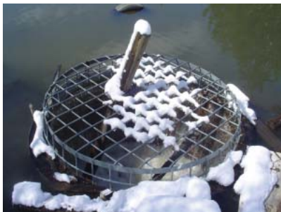
Typical vertical CMP with trash rack, Eloise Basin during snowmelt WY04
