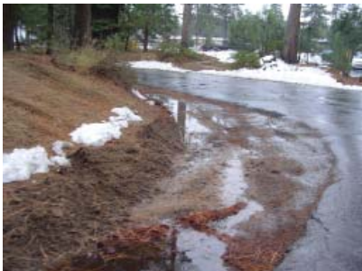
Example of roadside erosion in South Lake Tahoe, CA
